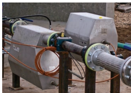
The WPS facility utilizes Actaris dual-tube mass flow meters for both liquid and vapor measurement. Shown above is a 3-in. m300 unit (left) for liquid; at right is an m200 unit for vapor.
